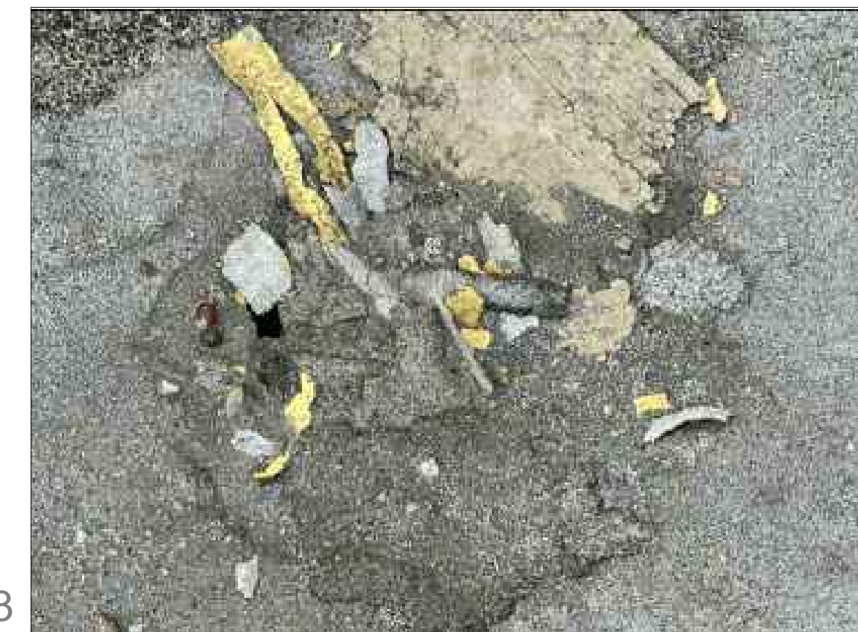
EXISTING CORROSION CAUSED BY THREE EXHAUST PIPES AT EAST FACADE
