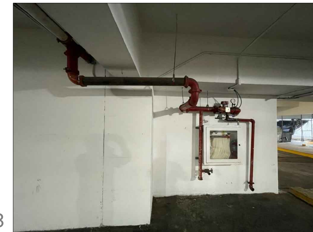
EXISTING FIRE CONTROLS SYSTEMS
