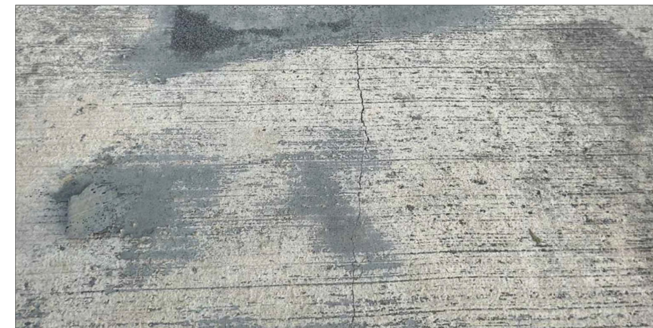
TYPICAL VIEW OF CRACKS
