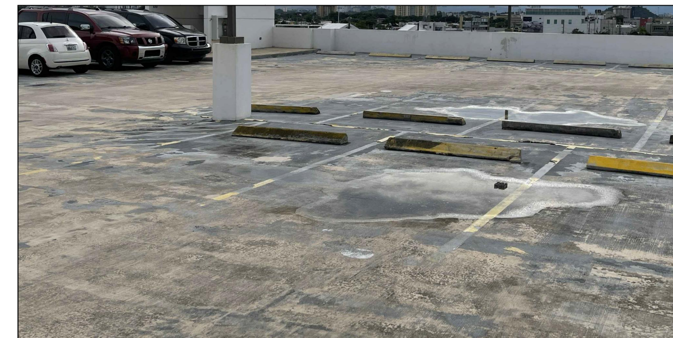
TYPICAL VIEW DRAINAGE PROBLEM
