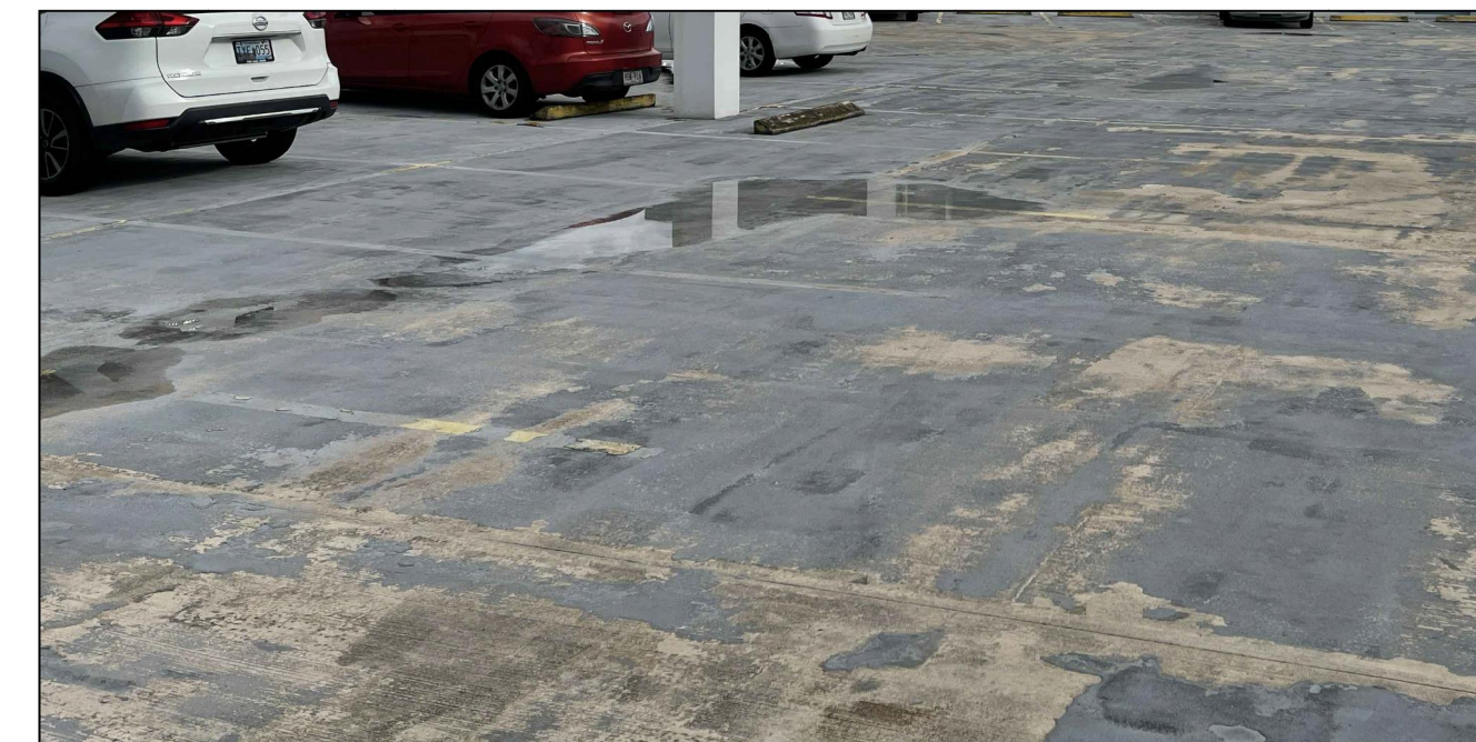
TYPICAL VIEW DRAINAGE PROBLEM
