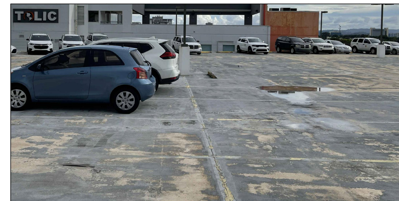
TYPICAL VIEW DRAINAGE PROBLEM
