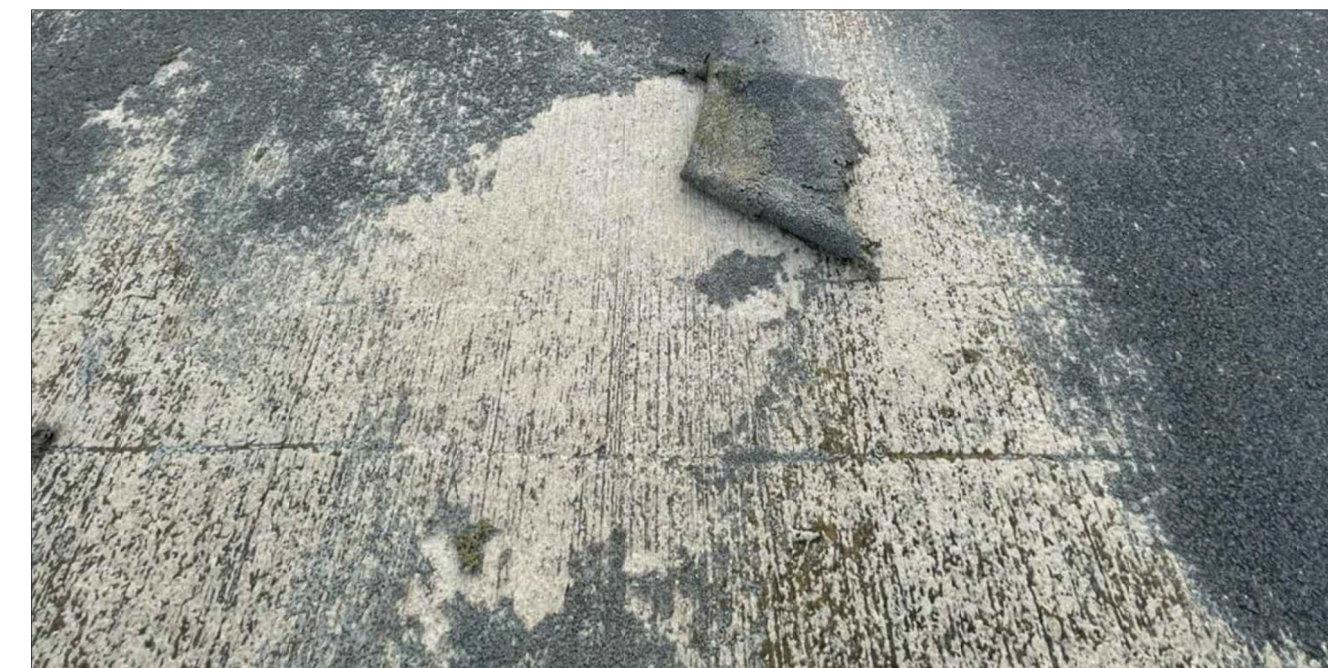
DAMAGE TRAFFIC SEALER SYSTEM
