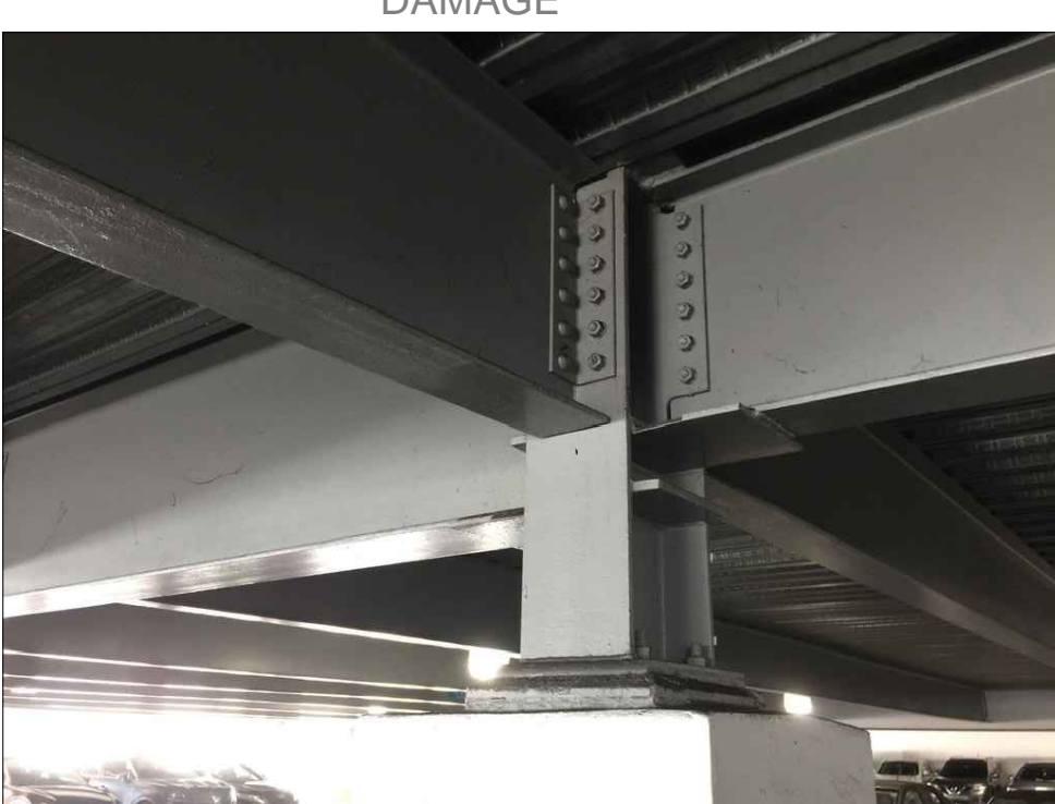
ELEMENTS WITH CORROSION AND PAINT DAMAGE
