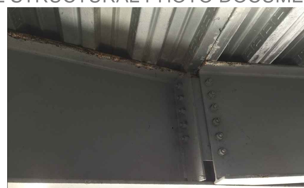
ELEMENTS WITH CORROSION AND PAINT DAMAGE
