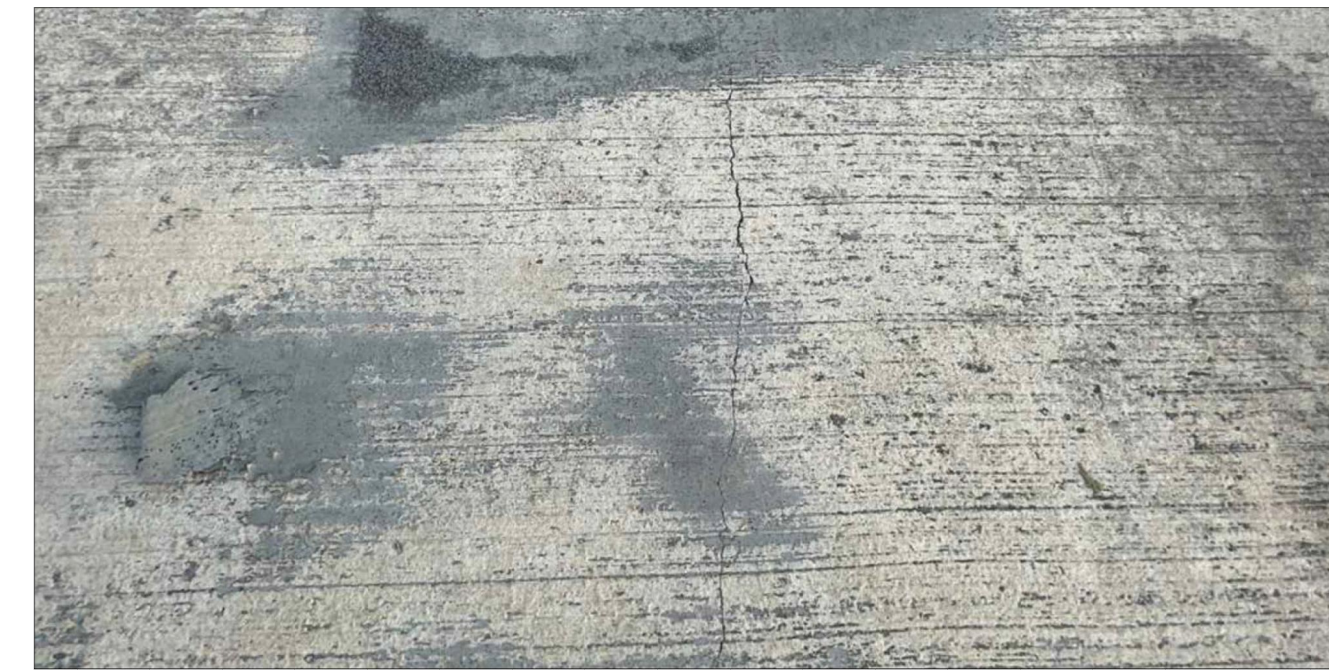
TYPICAL VIEW OF CRACKS
