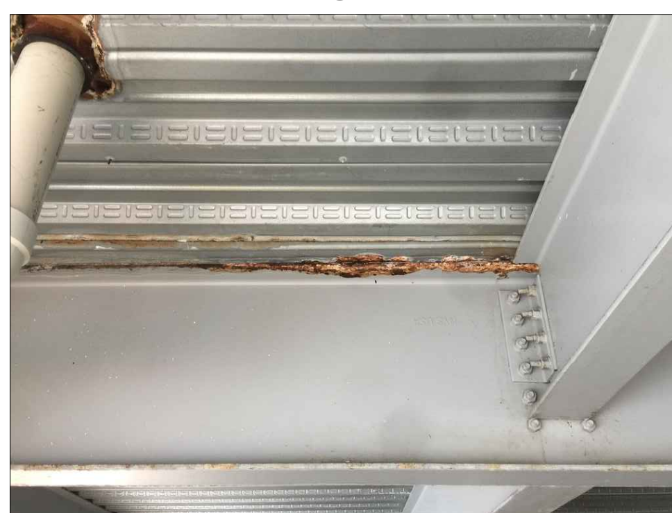
ELEMENTS WITH CORROSION AND PAINT DAMAGE
