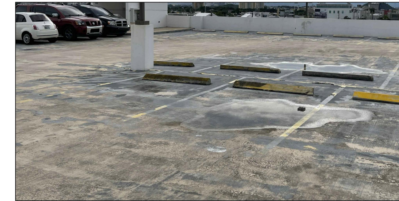
TYPICAL VIEW DRAINAGE PROBLEM
