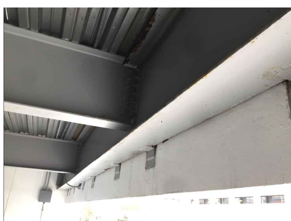
WATER INTRUSION BETWEEN CONCRETE PARAPET AND STEEL
