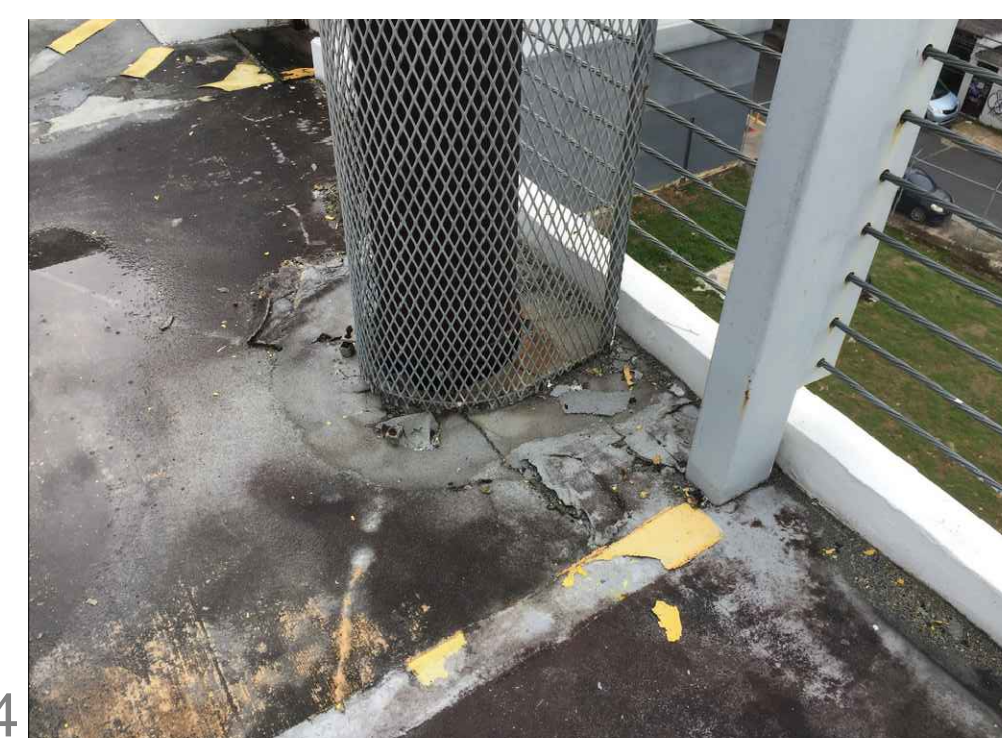
IMPROVEMENTS TO THE JOINT SYSTEM BETWEEN CONCRETE TILE AND THE GENERATOR EXHAUST SYSTEM
