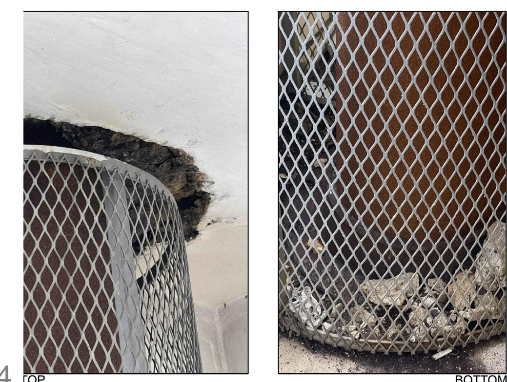
CORROSION CAUSED BY THREE EXHAUST PIPES AT EAST FACADE
