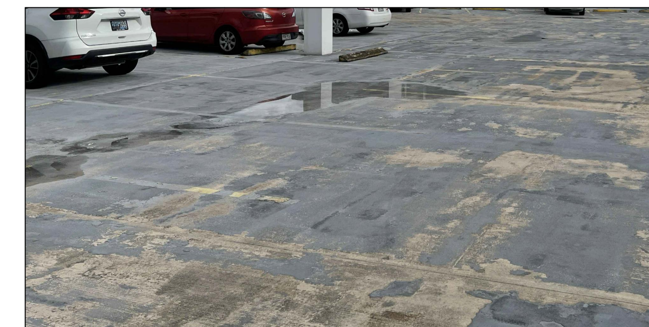
TYPICAL VIEW DRAINAGE PROBLEM
