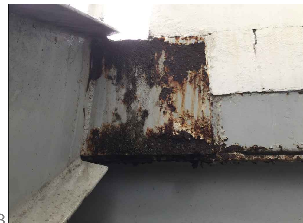
CORRODED STEEL ELEMENT
