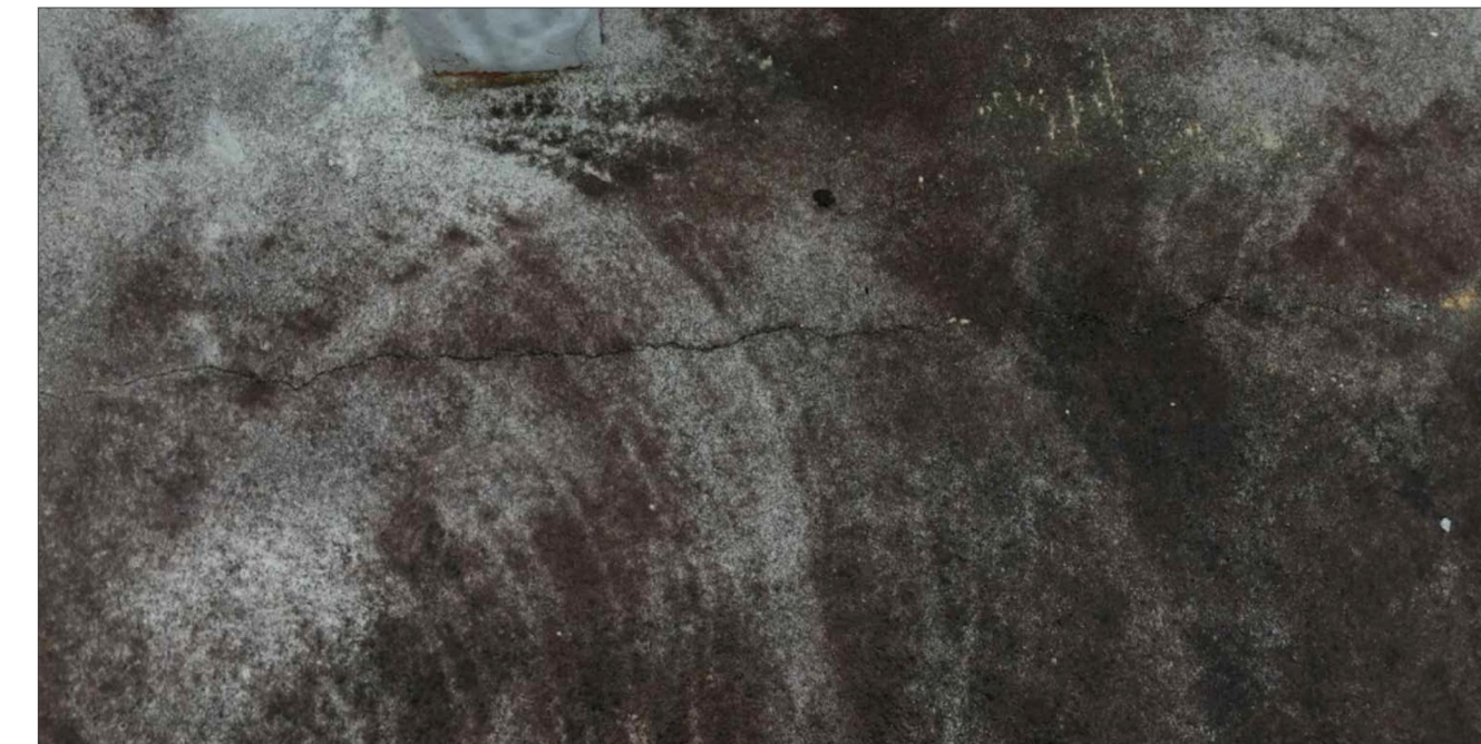
TYPICAL VIEW WATER PONDING AREA
