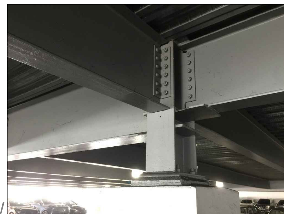
ELEMENTS WITH CORROSION AND PAINT DAMAGE
