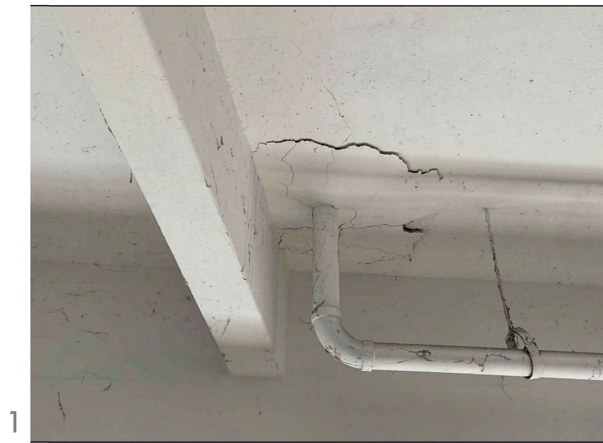
CORROSION OF CONCRETE SLAB AT CORNER
