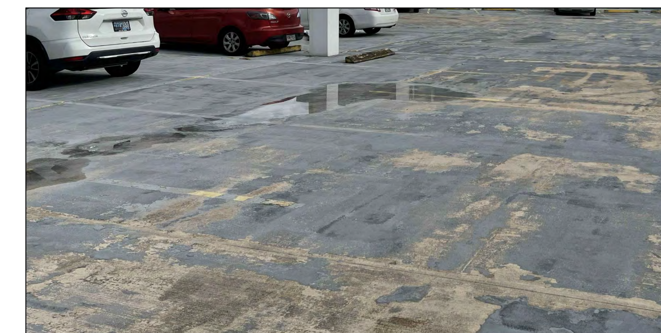
TYPICAL VIEW DRAINAGE PROBLEM
