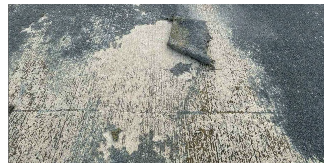
DAMAGE TRAFFIC SEALER SYSTEM
