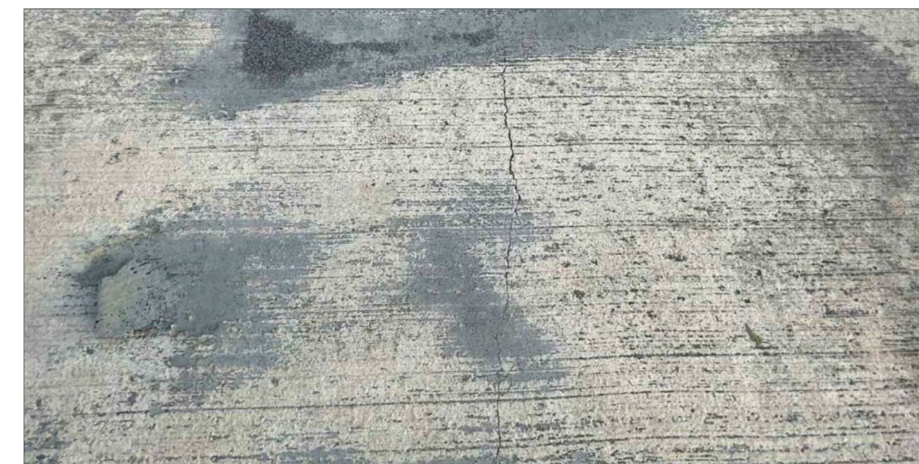
TYPICAL VIEW OF CRACKS
