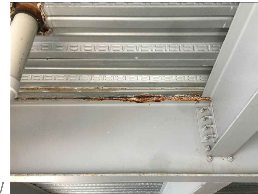
ELEMENTS WITH CORROSION AND PAINT DAMAGE
