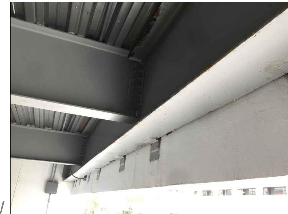
WATER INTRUSION BETWEEN STEEL CONCRETE PARAPET AND STEEL
