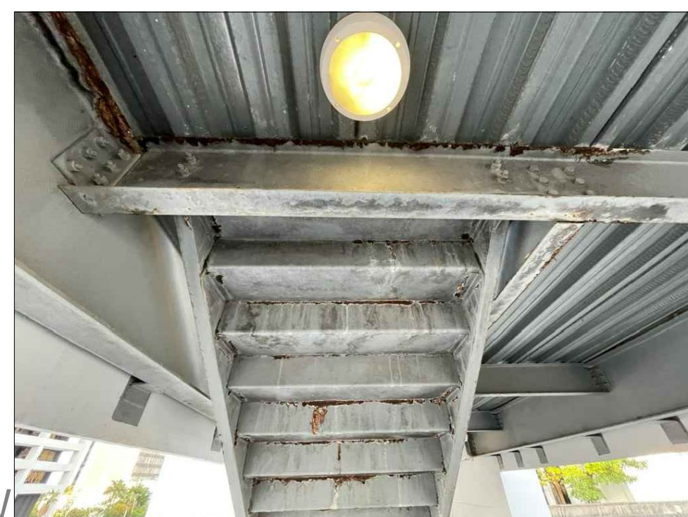
ELEMENTS WITH CORROSION AND PAINT DAMAGE
