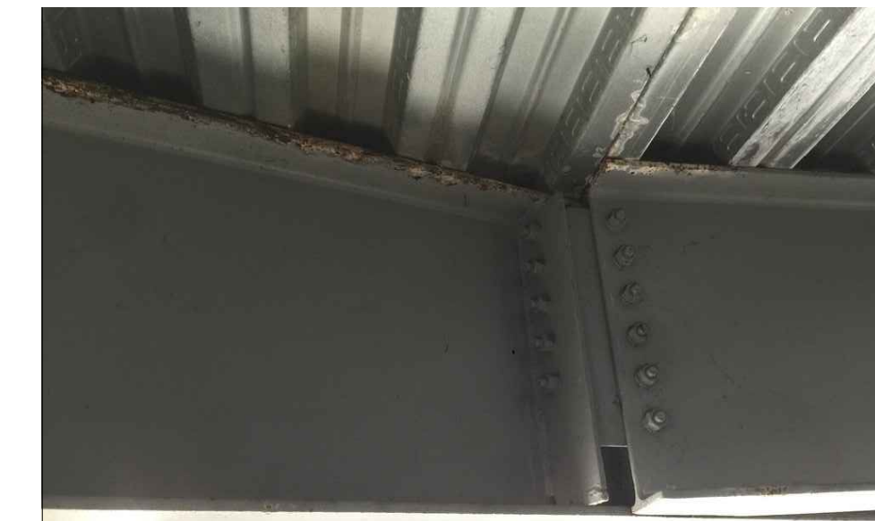
ELEMENTS WITH CORROSION AND PAINT DAMAGE
