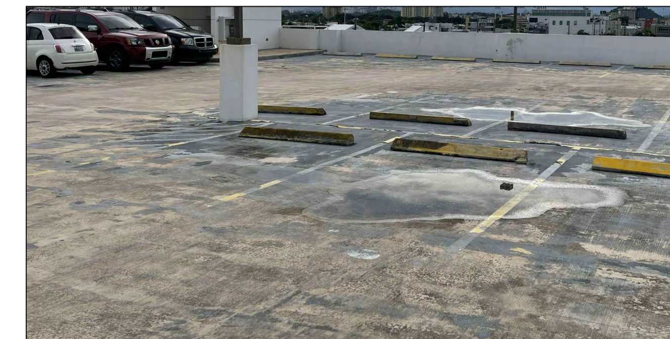
TYPICAL VIEW DRAINAGE PROBLEM
