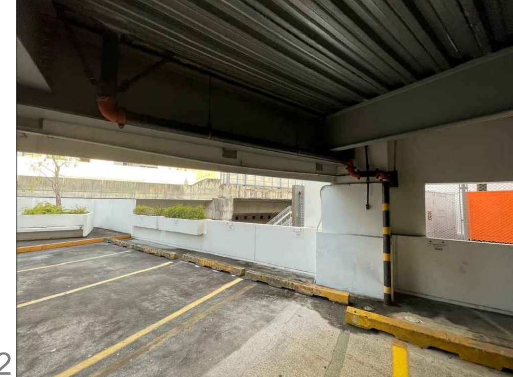
FIRE CONTROLS SYSTEMS TO BE PAINTED
