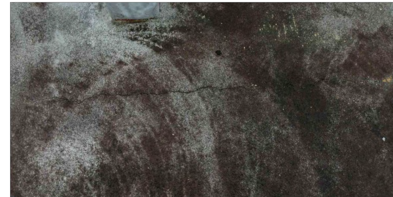
TYPICAL VIEW WATER POUNDING AREA
