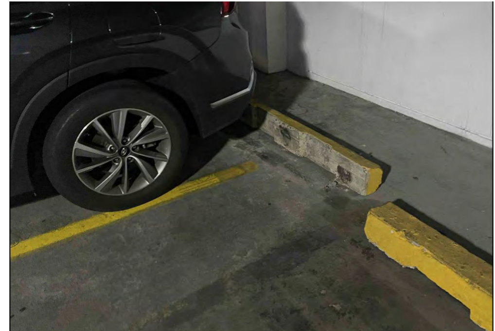
WHEEL-STOPS WITH INADEQUATE SUPPORT
