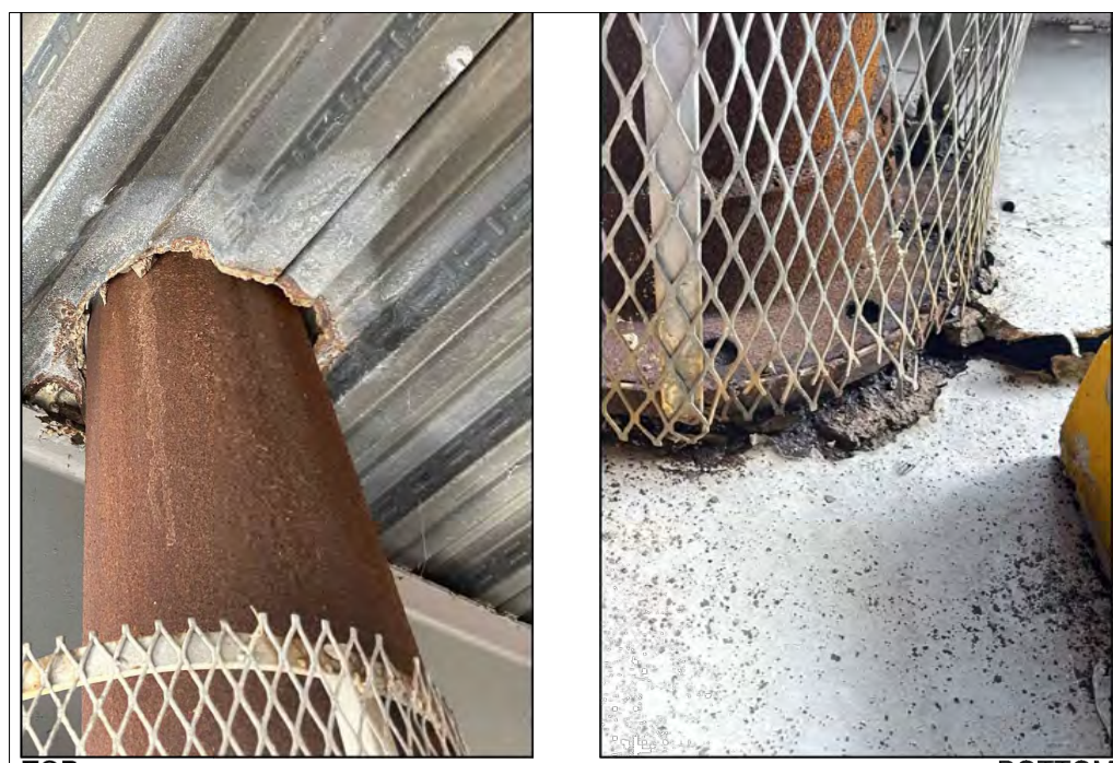
CORROSION CAUSED BY THREE EXHAUST PIPES AT EAST FACADE
