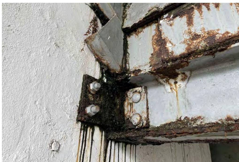
CORROSION OF BEAMS OF STAIR AT SOUTH-WEST STAIR
