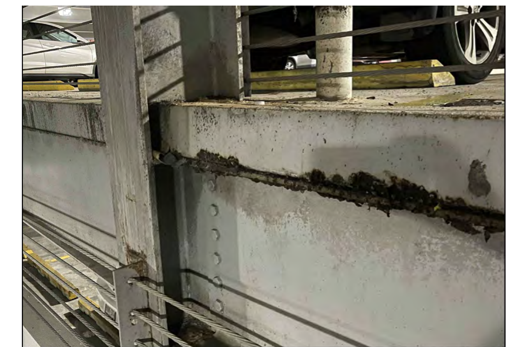
CORROSION OF BEAMS AND METAL DECK ALONG LONGITUDINAL AXES OF THE RAMPS
